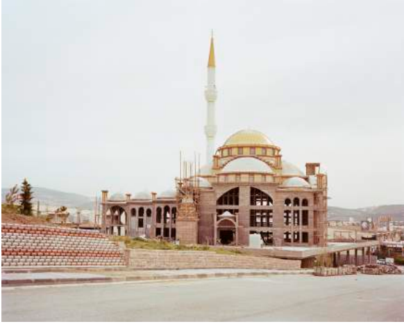
NORMAN BEHRENDT İVEDİK YAVUZ SULTAN SELİM CAMI, UNDER CONSTRUCTION, YENİMAHALLE, ANKARA 2016, FROM THE BRAVE NEW TURKEY SERIES. COURTESY OF UNO ART SPACE/ HARTMANN PROJECTS, STUTTGART.
