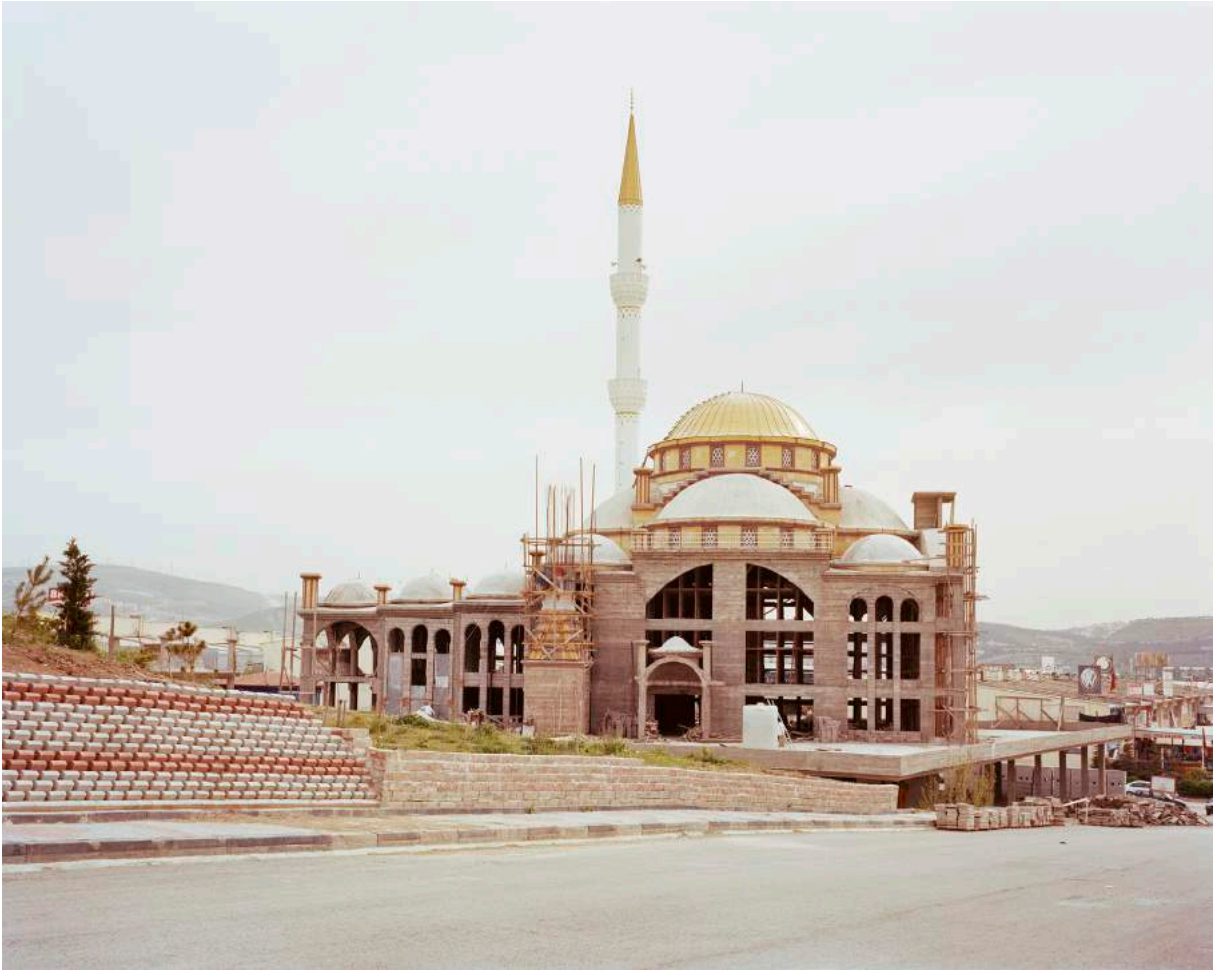
NORMAN BEHRENDT İVEDİK YAVUZ SULTAN SELİM CAMI, UNDER CONSTRUCTION, YENİMAHALLE, ANKARA 2016, FROM THE BRAVE NEW TURKEY SERIES.
